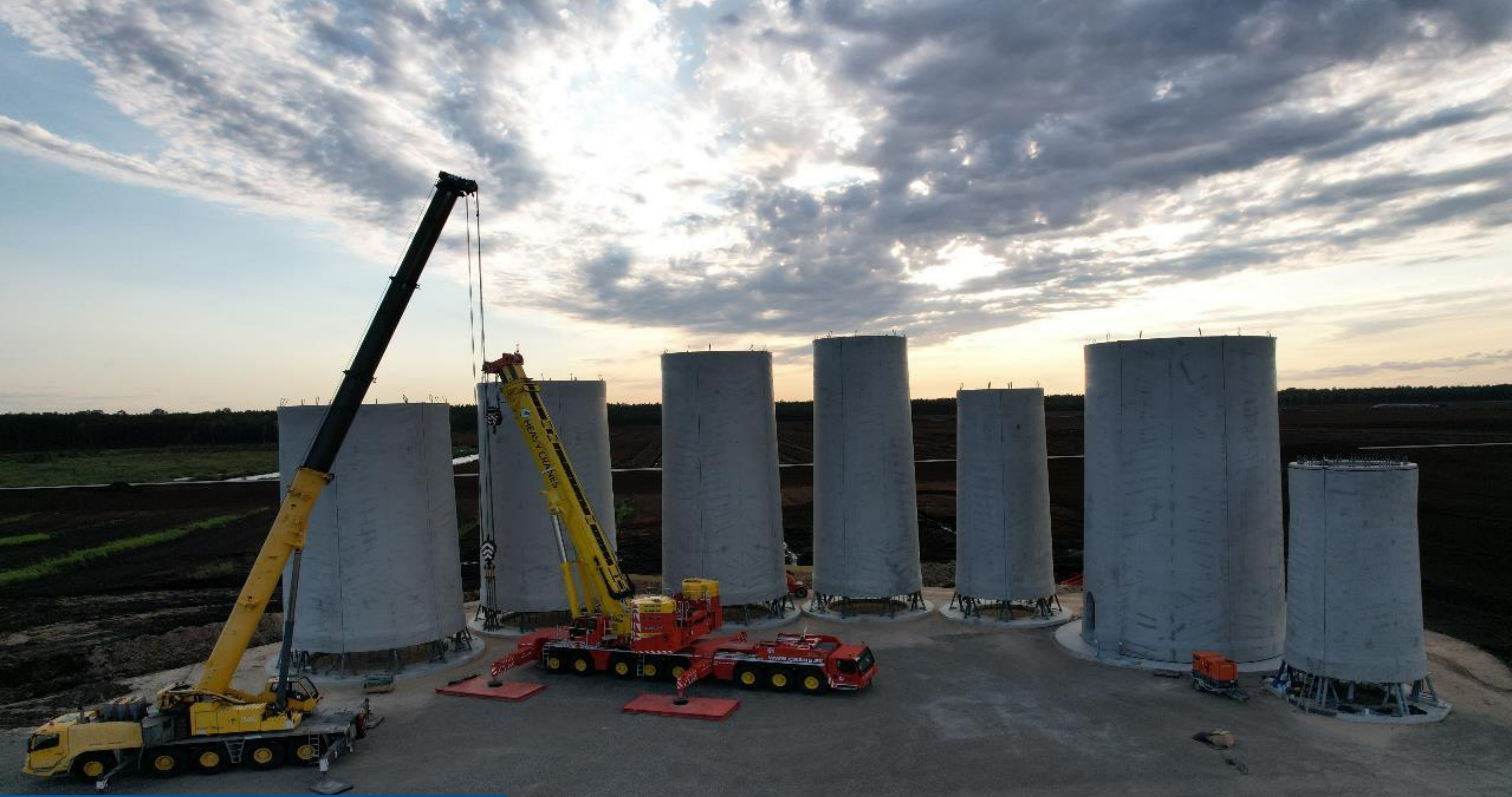
2. Laflora Energy / 108.8MW
